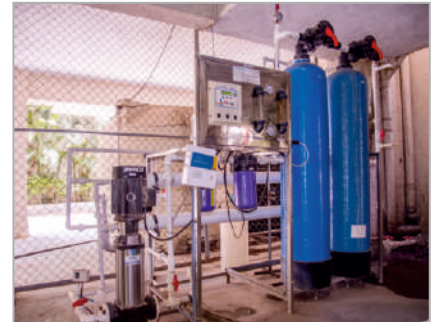
RO Plant for Drinking Water
