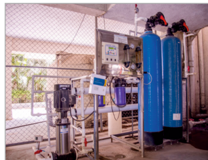
RO Plant for Drinking Water
